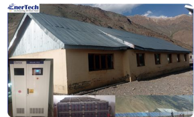
Application: Micro Grid Rating: 100kW/200kWh Site location: Ladakh, India
