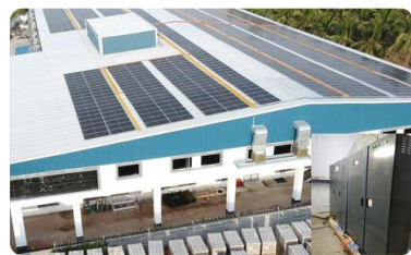
Application: Cold Storage Rating: 300kW/400kWh Site location: Kanpur, India
